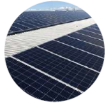
Solar PV Panels
