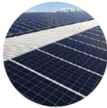
Solar PV Panels
